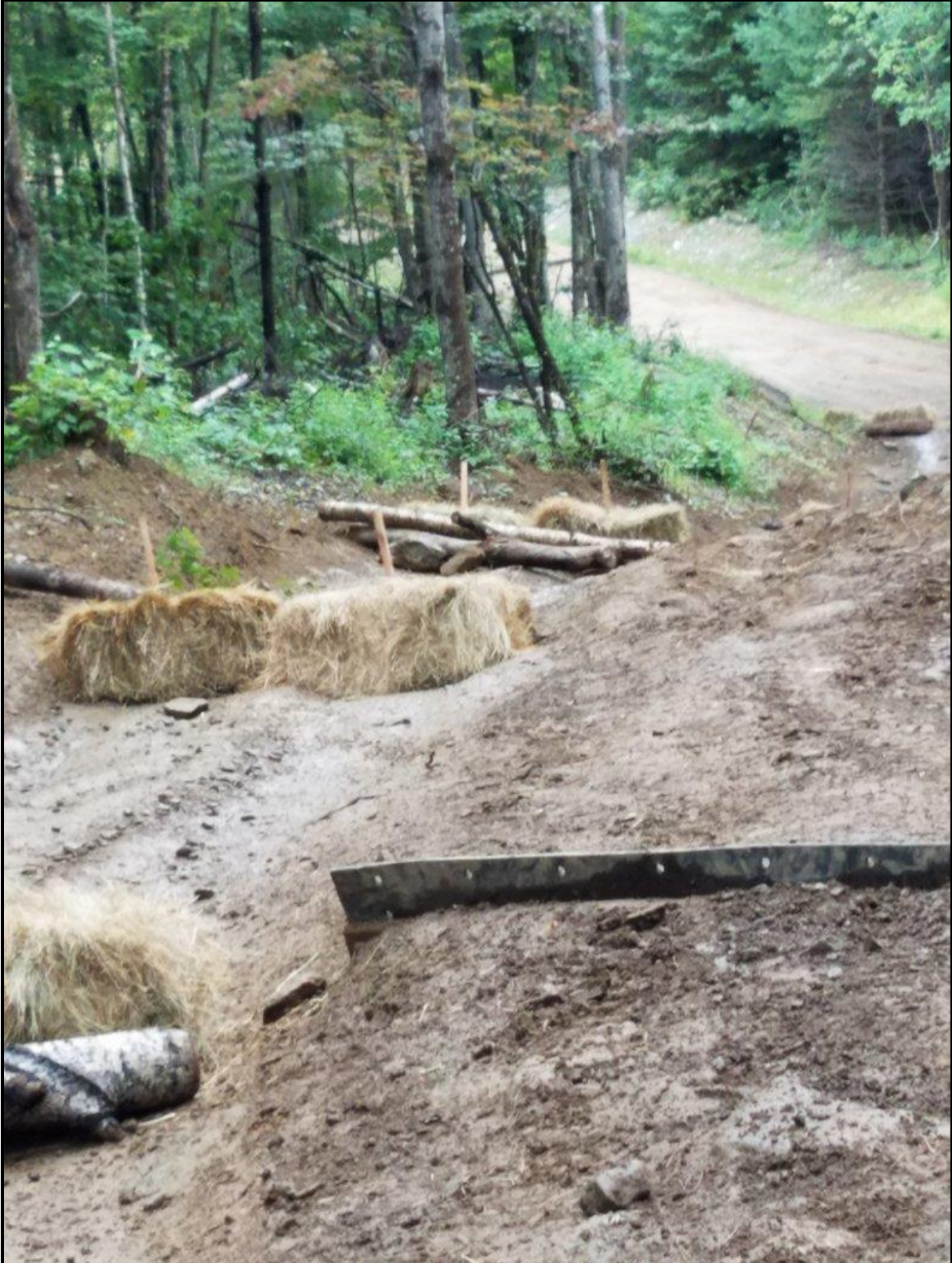
Hay bales with stakes through them and logs in front discourage riders from riding up the sides of the trail creating erosion and washouts.
