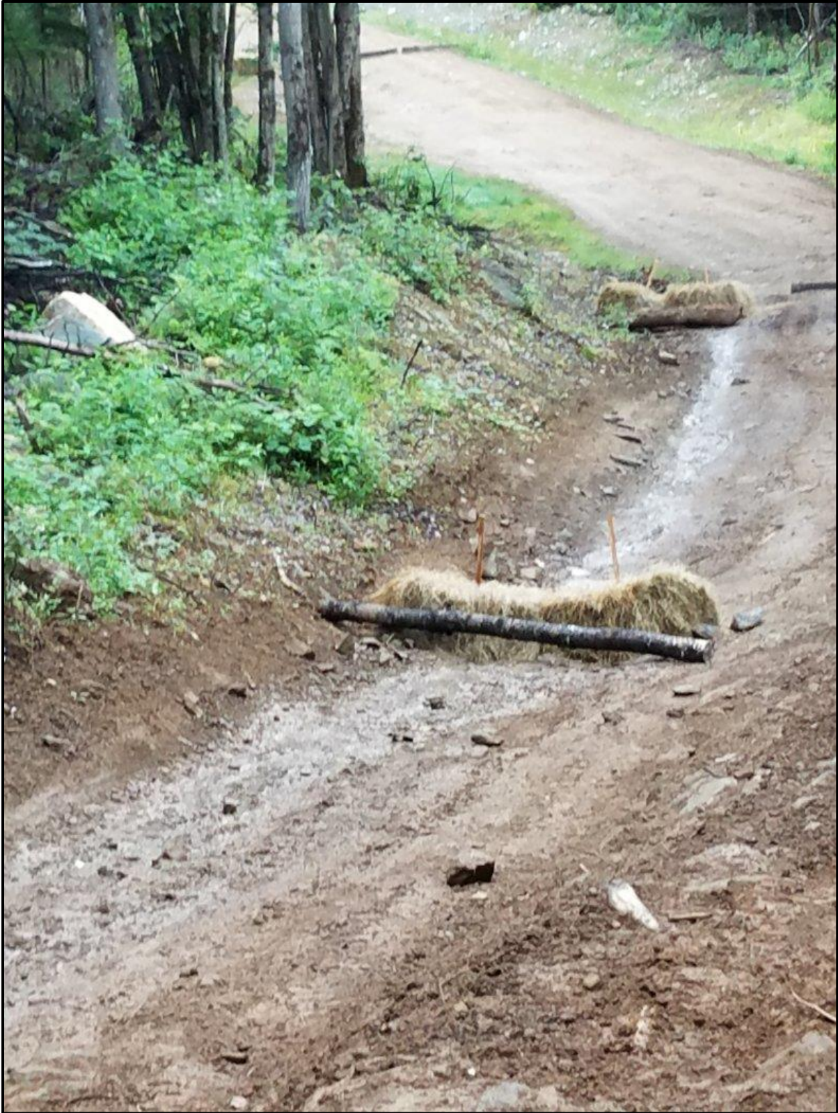
A total of 50 hay bales were installed along a half-mile of trail.
