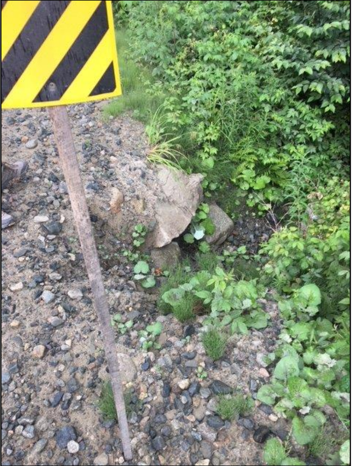
Washout about a mile south of Rt. 110B gate.
