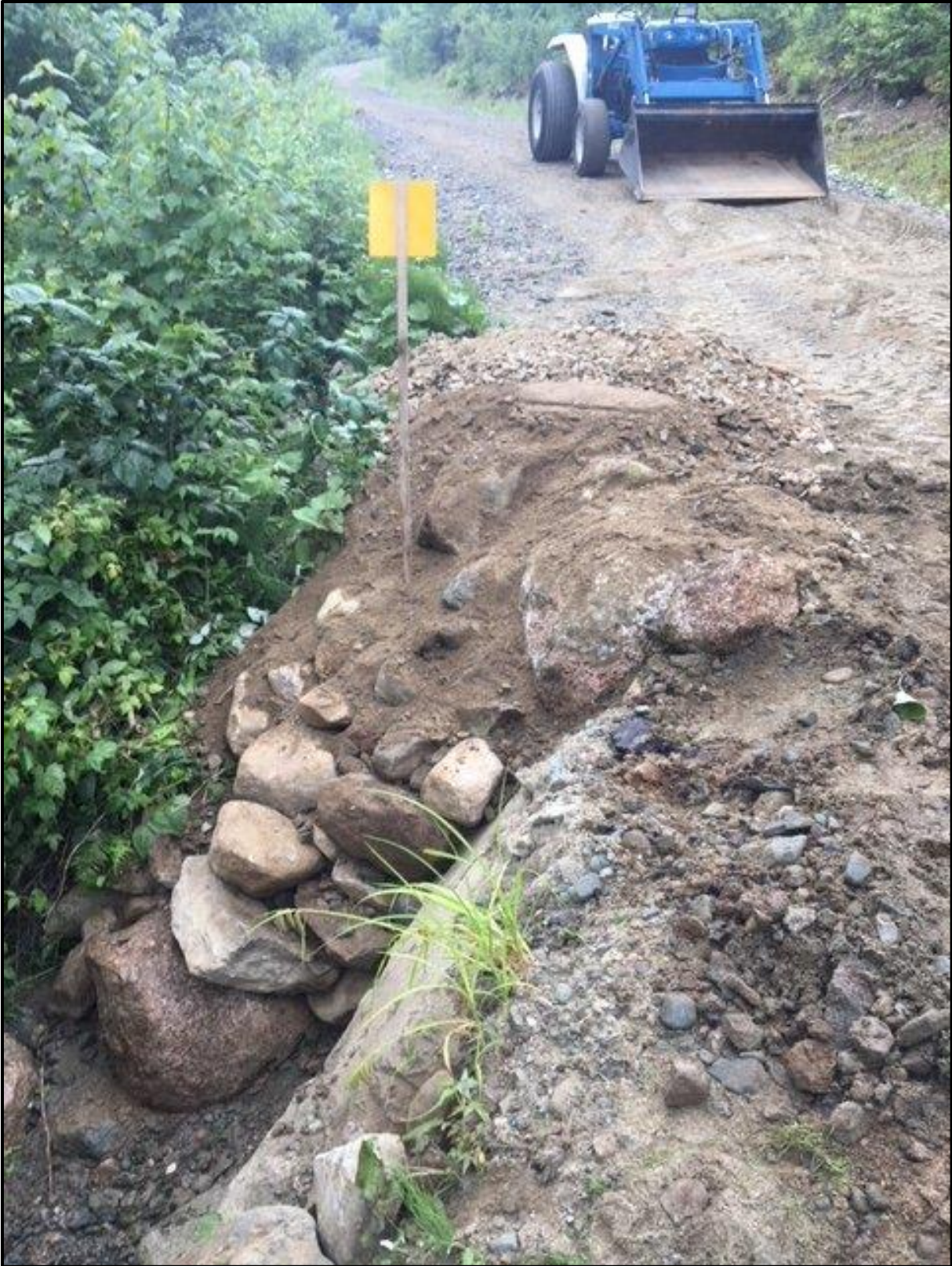
Completed washout repair with gravel on top of stacked rocks. Andy's tractor is in the background.
