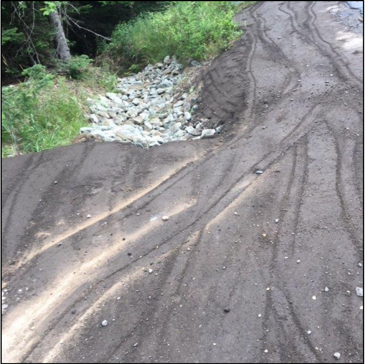
Picture of the Rt. 110B washout after it was fixed by NH DOT crews.
