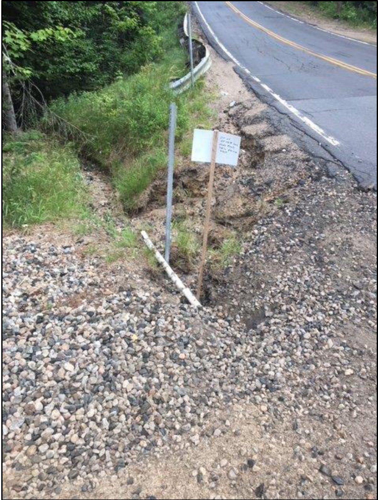
Washout where the Head Pond Connector Trail connects with Rt. 110B.
