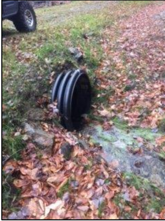
The extra-large 36" culvert donated by the NH ATV Club is doing its job.
