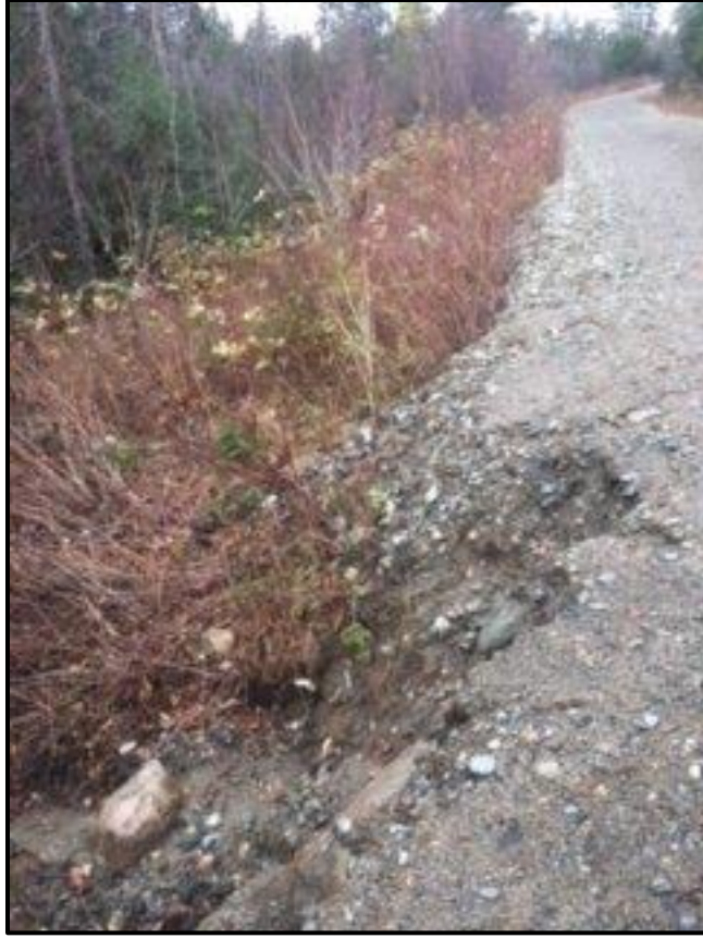
One small washout on the existing gravel road leading up to Rt. 110B. This will be easily fixed next spring before the trail opens.
